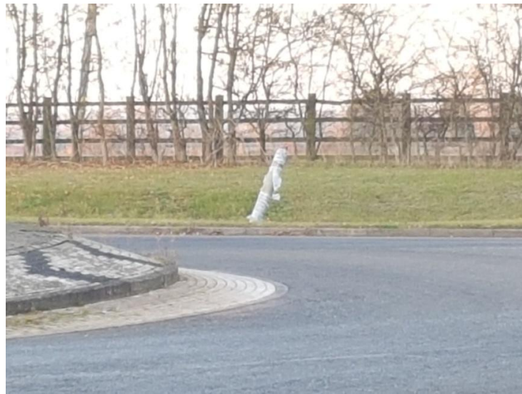
Photo 3.2.1 Damaged lamp column
