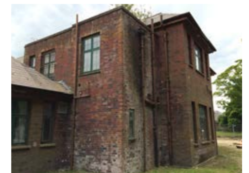
Damp structure to be demolished
