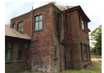
Damp structure to be demolished
