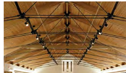
Glulam timber with slender steel bracing
