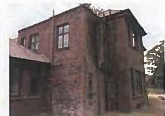
Damp structure to be demolished
