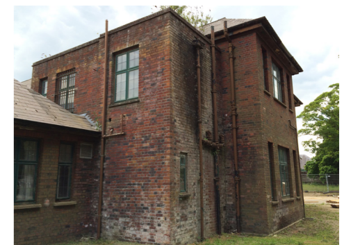
Damp structure to be demolished
