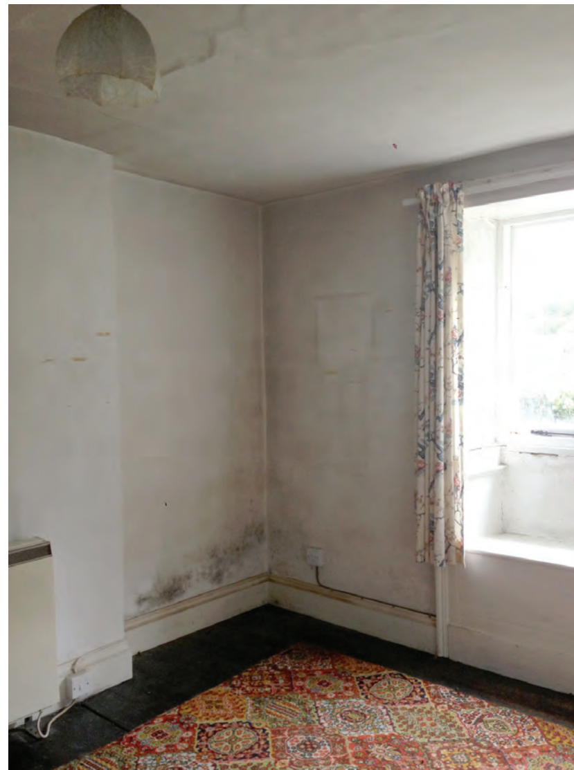
Fig.27 - Dining room - damp
