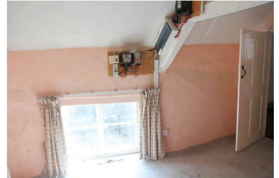
Fig.26 - Bedroom 2 - electrical incoming mains and distribution boards
