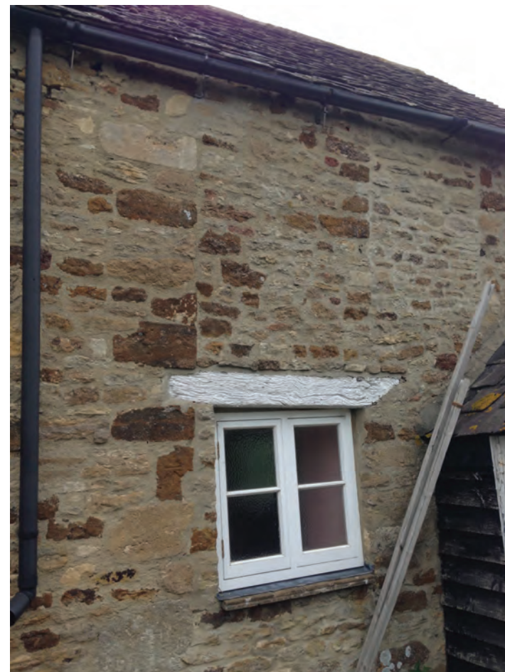
Fig.20 - Line down stonework
