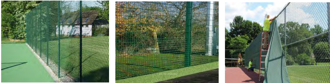
Illustrative court perimeter fence types including the use of additional ‘wind break’ detail on exposed site
