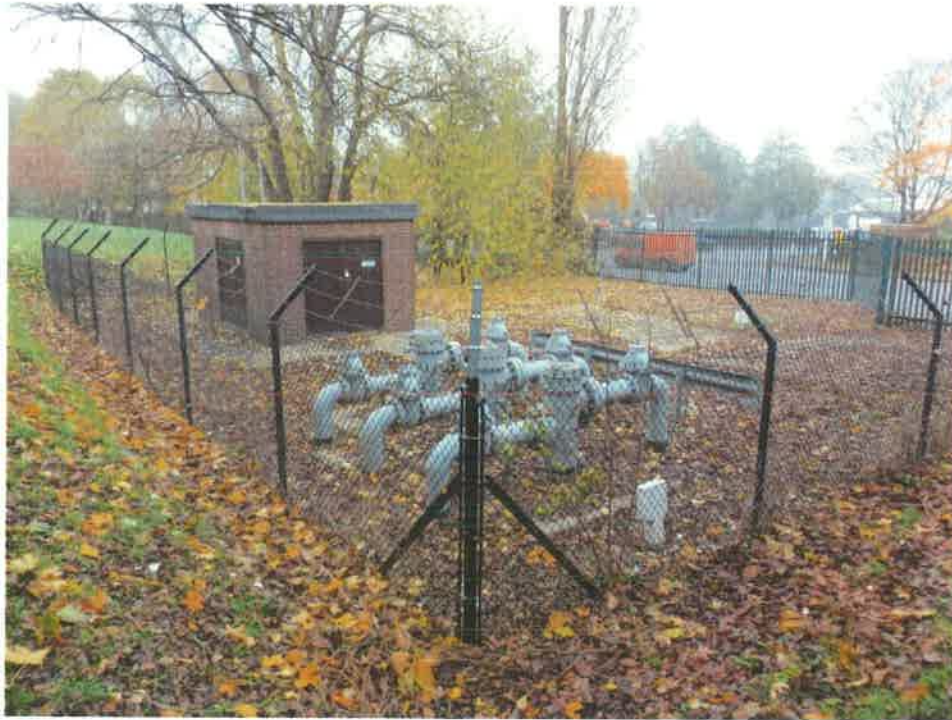
Photo 9: View towards gas infrastructure station located outside the eastern site boundary, looking north-east from eastern site boundary. The station is located on a small, square cut platform at a lower level than the study site in this area.
