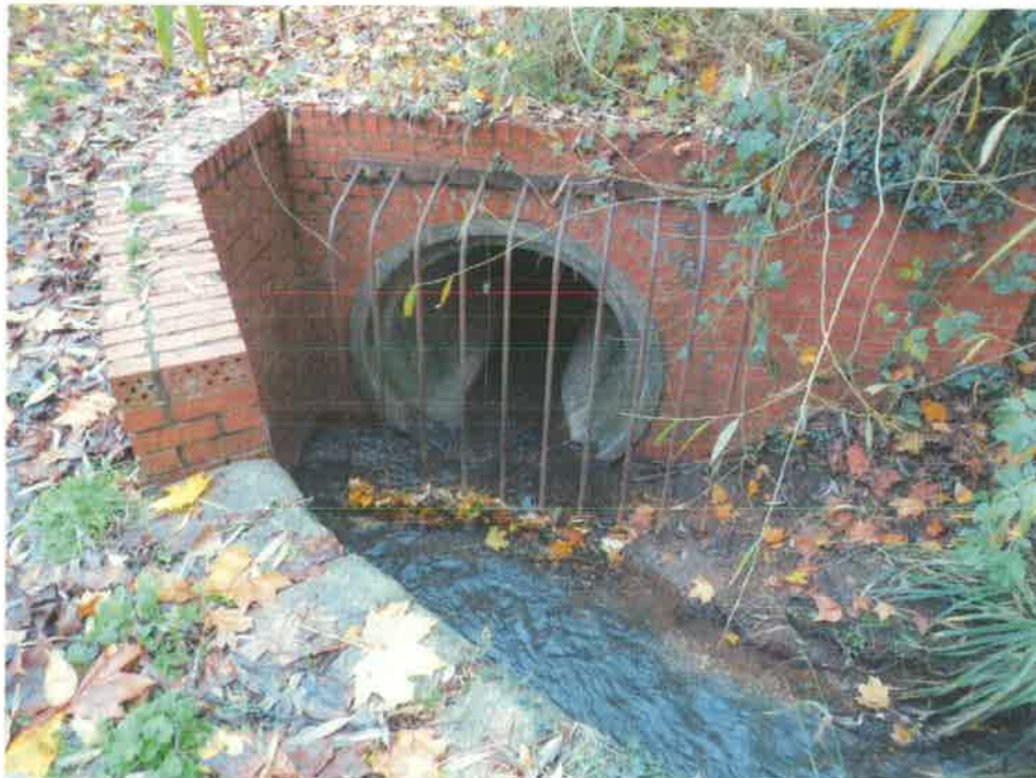
Photo 10: View of Birds Brook as it diverts in a southerly direction into a culvert which runs down the eastern site boundary, looking south from the eastern site boundary.
