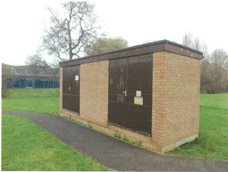
Photo 5: View of gas infrastructure installation located on the western site boundary, looking north-east.
