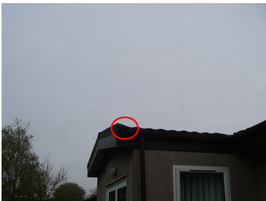
Photograph 3: Small section of lifted felt offering some limited roosting opportunities for bats.
