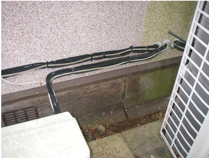
Photograph 4: A mammal burrow beneath building B1 on the eastern building aspect.
