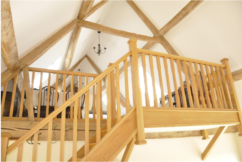
The roof structure of the northern barn with a replacement roof structure. Apart from the stone ventilators, there are no historic features remaining.
