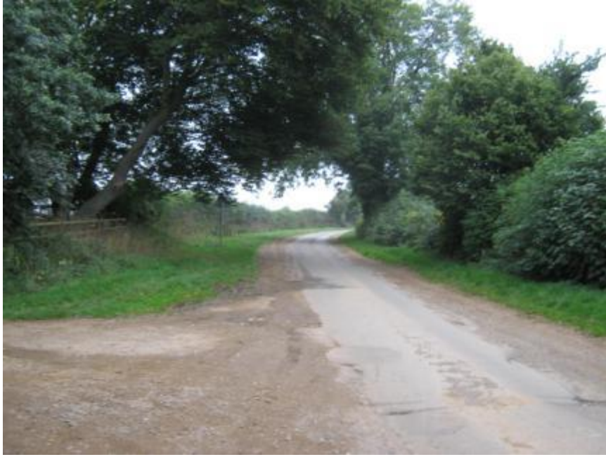
View of the damage in Grange Lane
