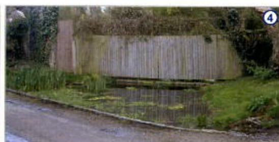
Balancing pond as part of a sustainable drainage system.
