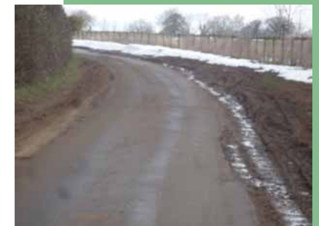
Significant Erosion to Lane Edges
