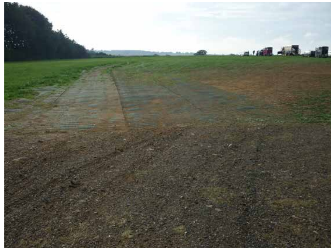
Ground reinforcement to reduce traffic wear on the access to the site
