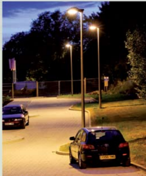
Column and/or bollard lighting to car park (30lux)
