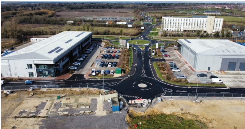
FIG 22- DRONE PHOTOGRAPH DOWN CATALYST ESTATE ROAD AND CHARLES SHOULER WAY SHOWING CATALYST PHASE 1 AND IHG HOLIDAY INN EXPRESS
