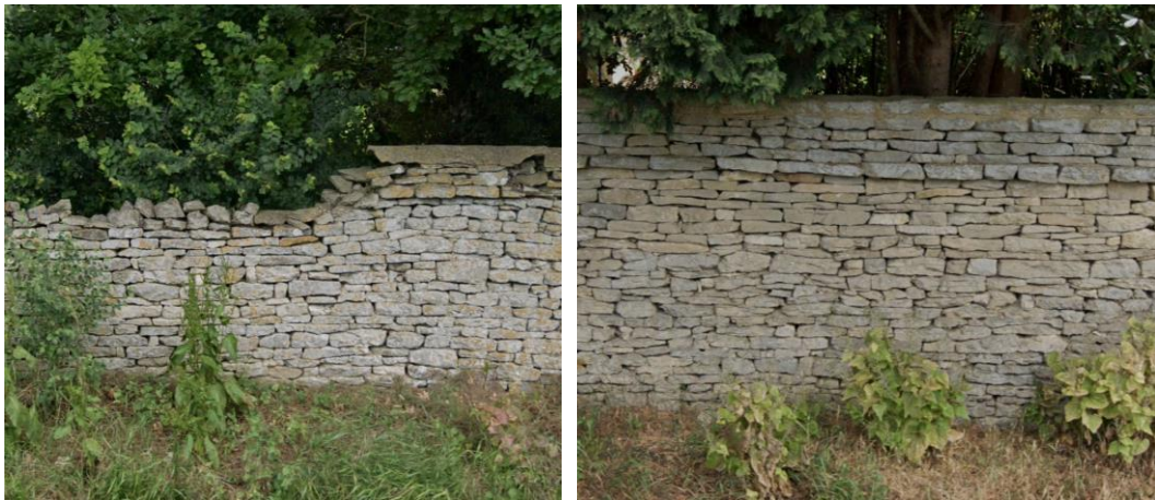
Figure 24 Areas of failed cement coping and dilapidating walling along Heyford Road; section of walling along Heyford Road repaired c.2011.
