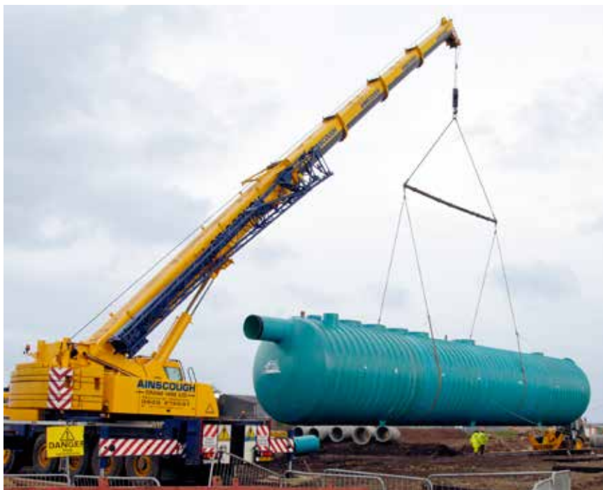
SPEL Puraceptor Class 1 full retention single chamber separator NS942 with 'automatic' Econoskim System serving a large catchment area (5.0 hectares) at Bristol International Airport.
