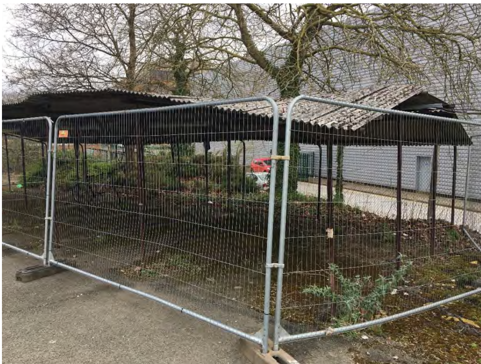
Photograph 44 – Fenced off bike shelter with possible asbestos containing materials.
