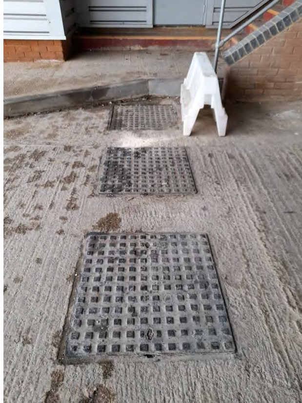
Photograph 17 – Potential Oil Interceptor in the south of warehouse area.
