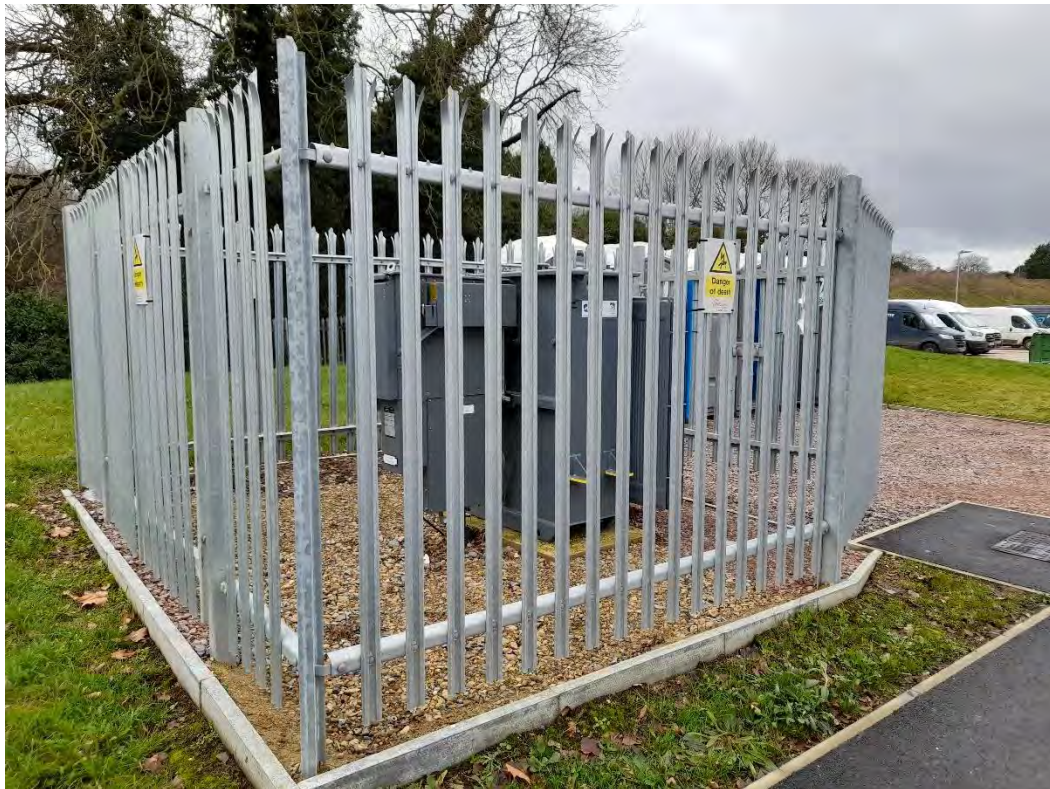
Photograph 22 – Electrical substation in south-west of the warehouse.
