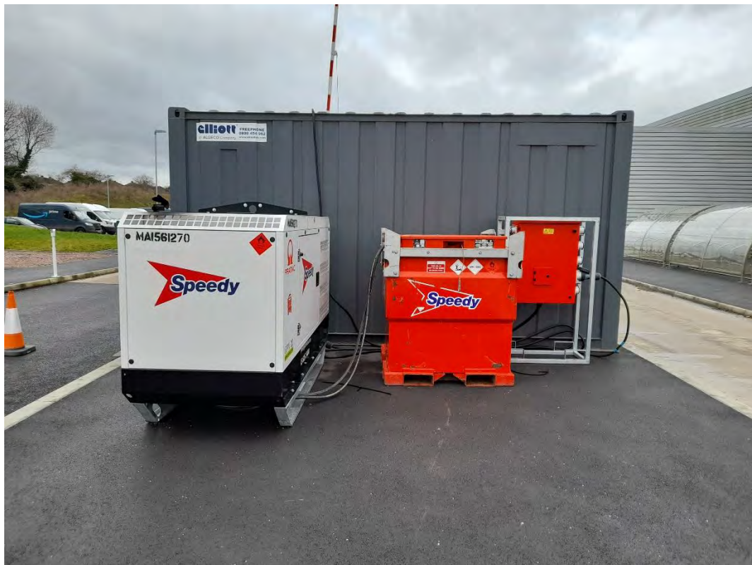
Photograph 24 – Generator and oil tank associated with hut.
