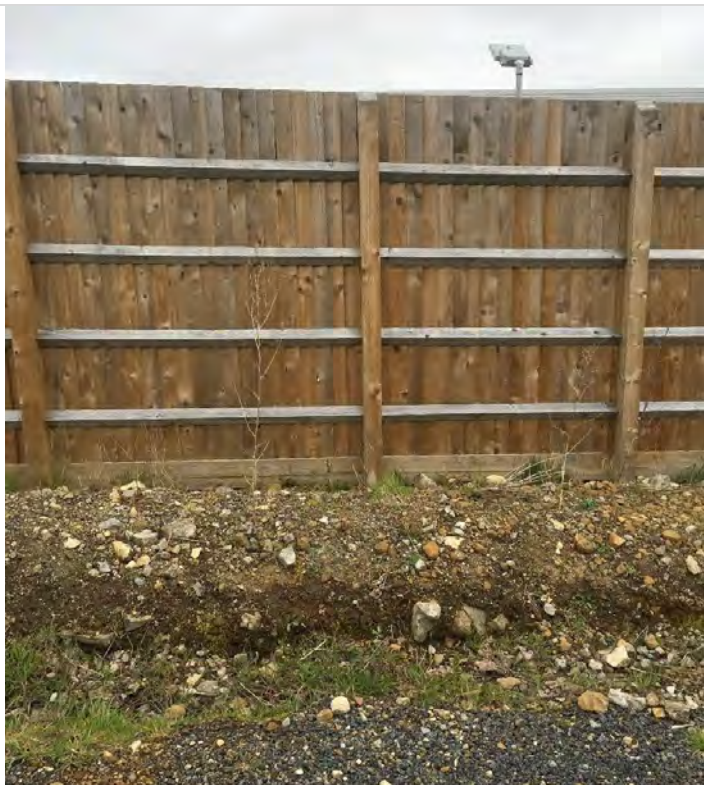
Photograph 34 – An informal trench with associated drainage along the eastern part of the car park.
