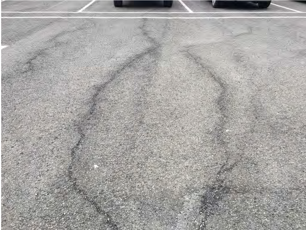
Photograph 33 – Wear in the asphalt surfacing.
