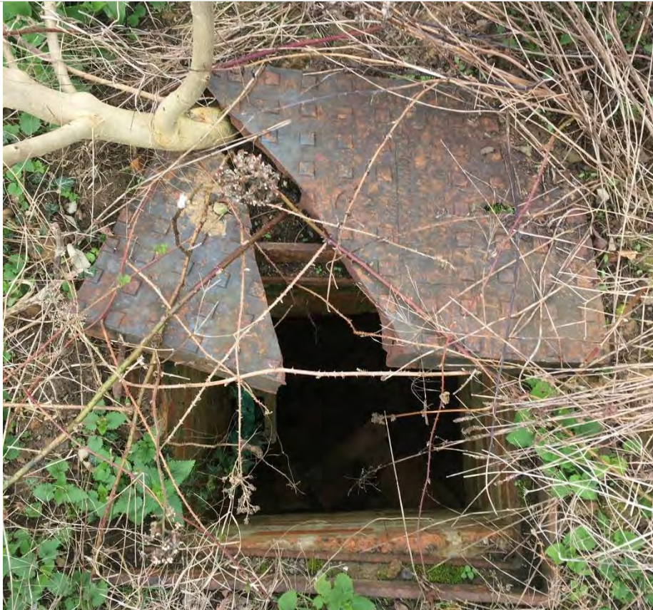
Photograph 46 – Damaged manhole cover in south-east of car park.
