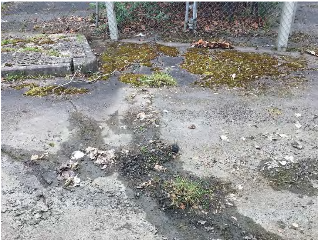
Photograph 32 – Cracks in asphalt possibly associated with nearby trees/vegetation.
