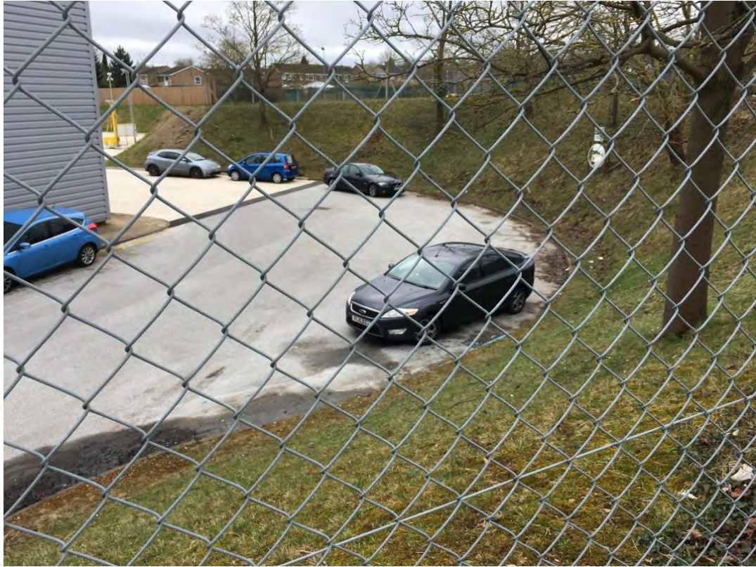
Photograph 43 – Vegetated retaining wall (approx. 4.5 m high); lower ground is the adjacent warehouse.
