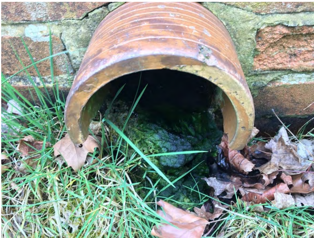
Photograph 38 – Pipe connecting to the stream with organic residue.
