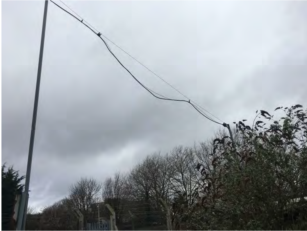
Photograph 41 – Overhead service from bike shelter to the small maintenance building.
