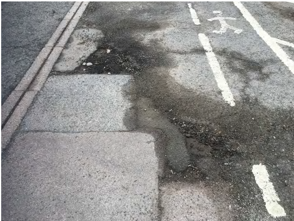
Photograph 30 – Asphalt with multiple patch repairs.
