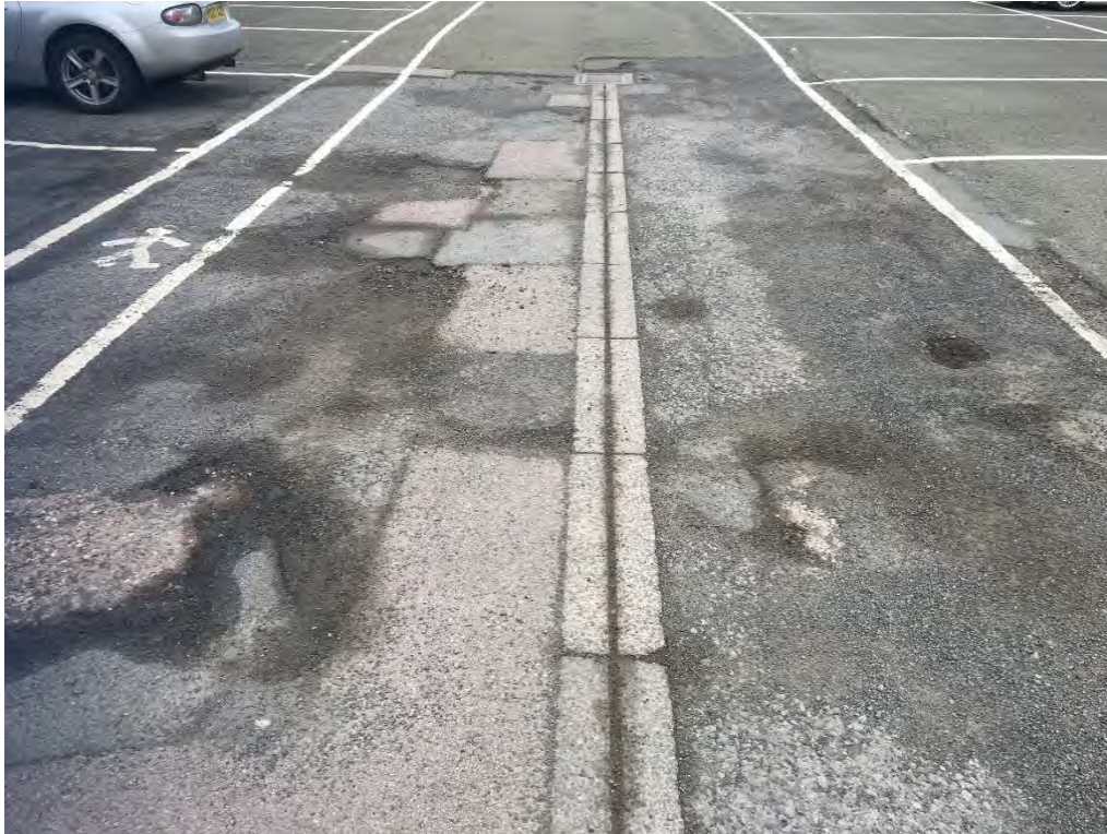
Photograph 31 – Evidence of wear and patch repair in asphalt surfacing in car park.
