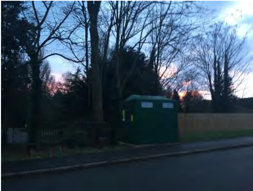
Photograph 13 – Substation in the south-eastern aspect of the Site
