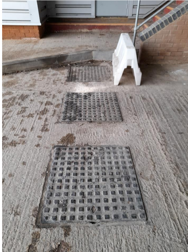
Photograph 17 – Potential Oil Interceptor in the south
