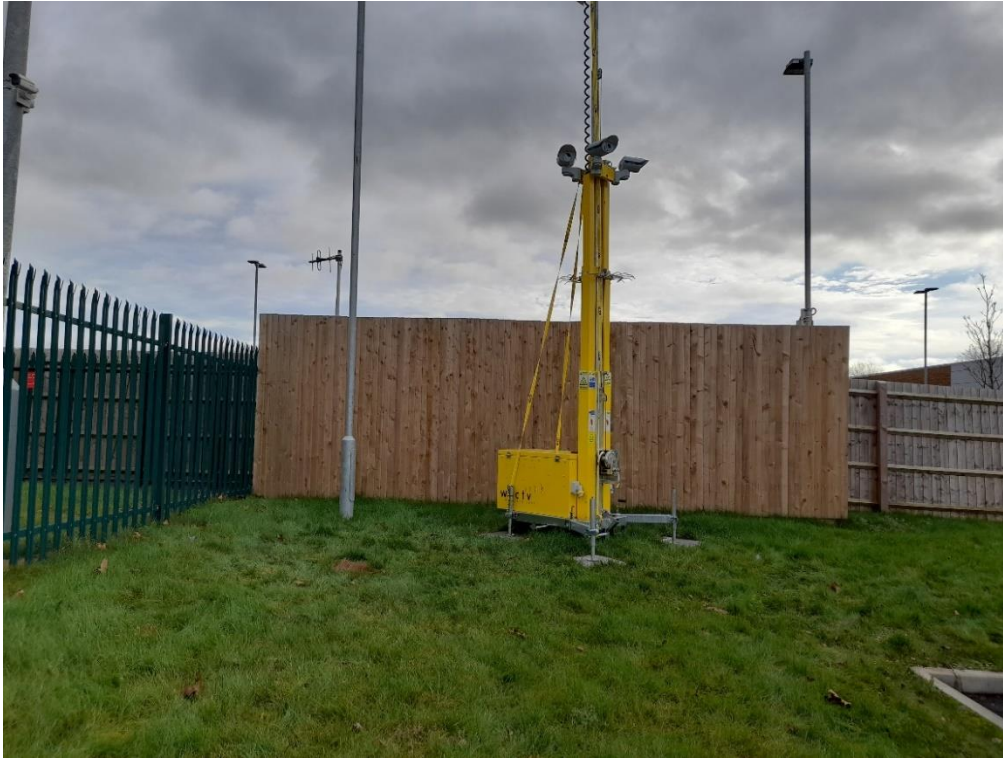
Photograph 7 – Substation with wooden enclosure in the north-eastern corner of the Site (outside of Site boundary)
