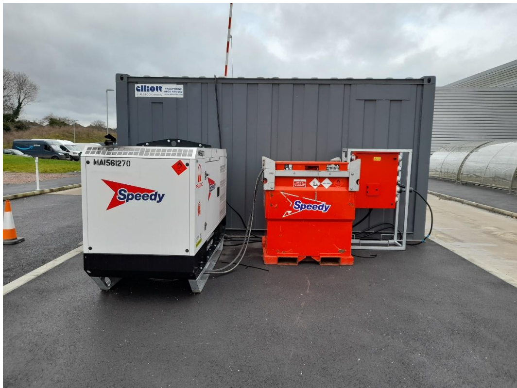
Photograph 24 – Generator and oil tank associated with hut
