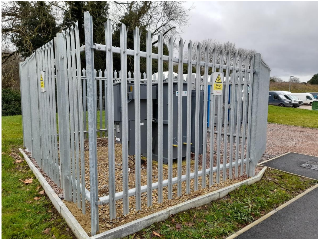
Photograph 22 – Electrical substation in south-west of the Site
