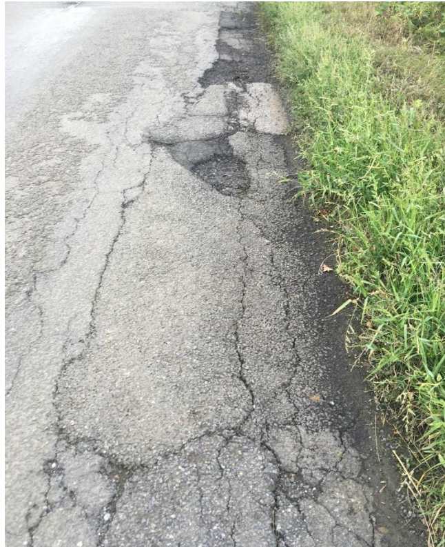
Figure 11 Overall Indicator of Pavement Risk “At Risk” Condition
